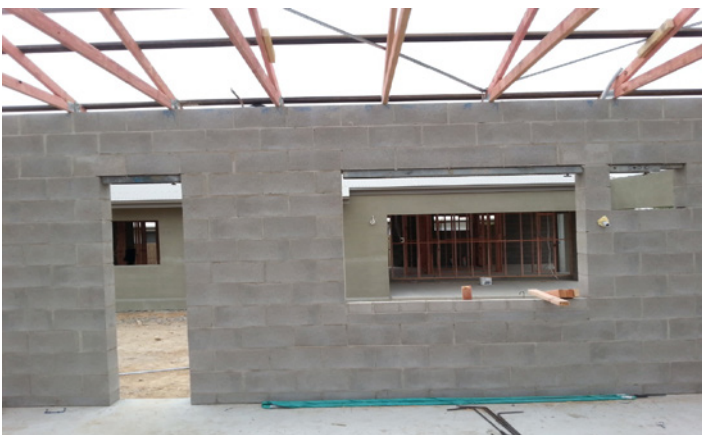
Trusses are anchored to the masonry wall, by a steel plate cleat which has the horizontal bond beam reinforcement threaded through it.
