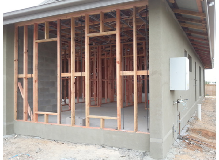
Threaded rod tie down anchors connect the timber wall frame to the slab which carries through and is fixed to the top plate.
